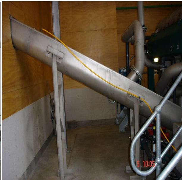
Figure 2: Sludge auger showing EM line plumbed into dewatered sludge auger
